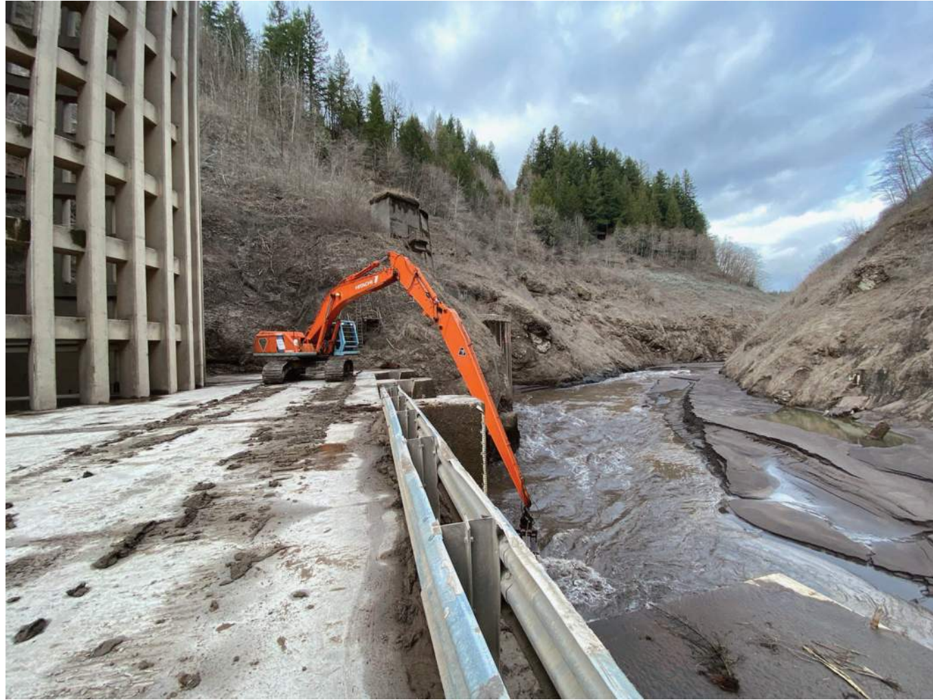
Picking LWD at the trash rack (pick the rack)
